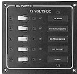
DC Circuit Breaker Panel
